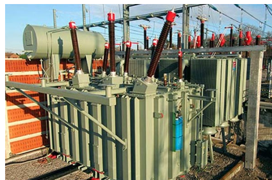
Phase-shifting transformer Source: Crompton Greaves
