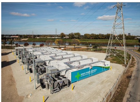
AES 40-MW battery in Dayton, Ohio Source: AES Energy Storage
